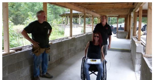
Bruce Duncan, Don Scott and Kristi McKechnie have made the office renovation possible.
