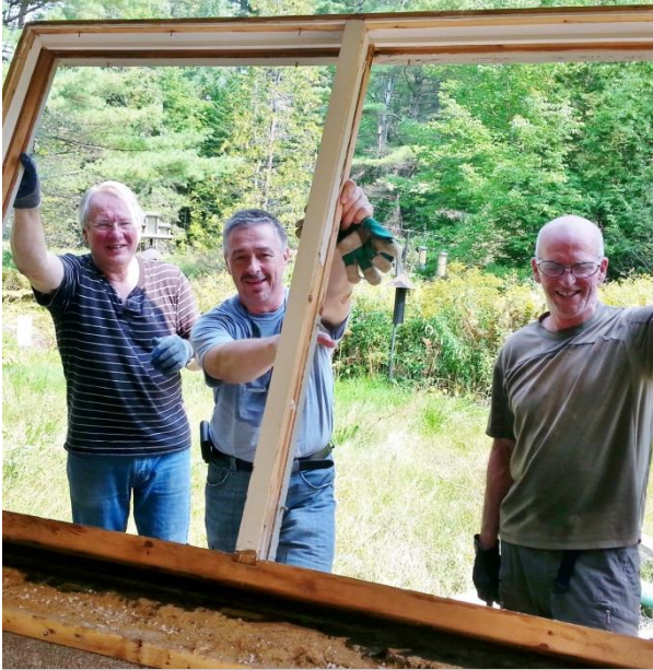
Volunteers Bruce, Hank & Kevin take out the old windows to make room for the new ones.
